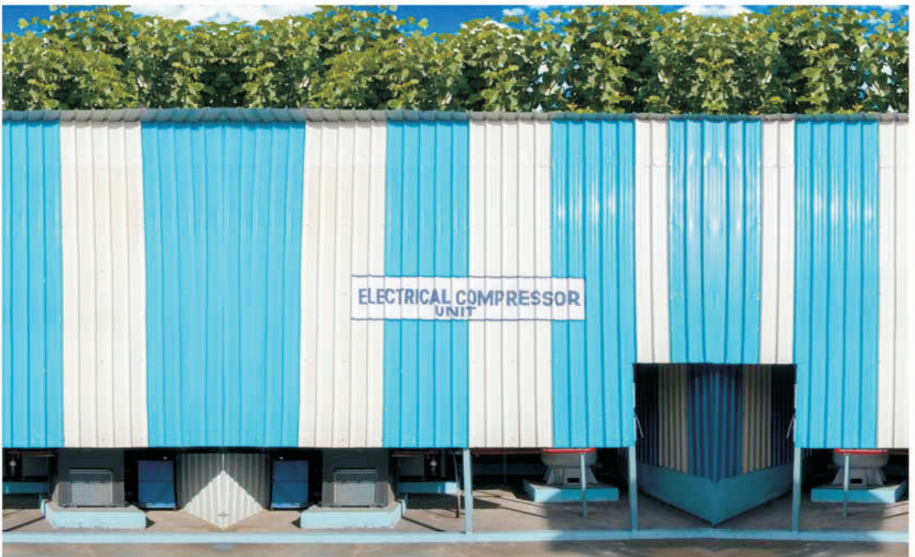
Electrical Compressor Unit (16 Bar - Pressure)
